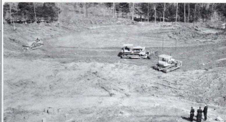
The surroundings take on a new face as bulldozers prepare the ground for the new wing.
